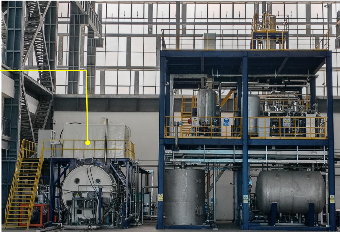
High heat flux testing facility & High pressure and temp. water loop
