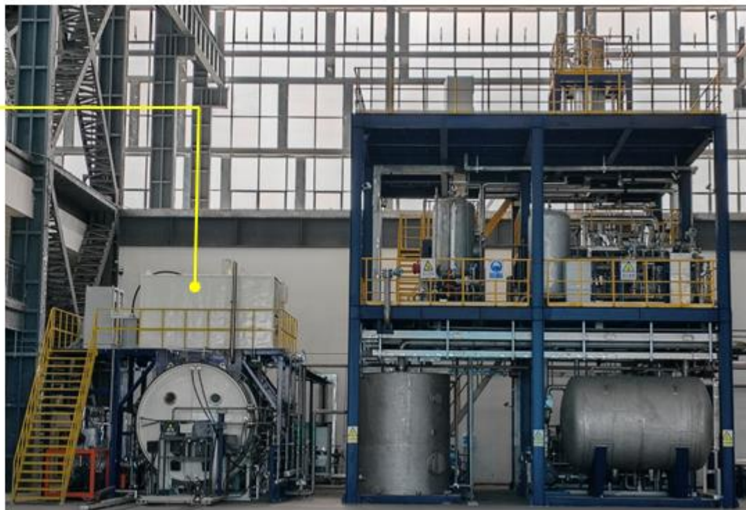
High temperature and high pressure water loop
