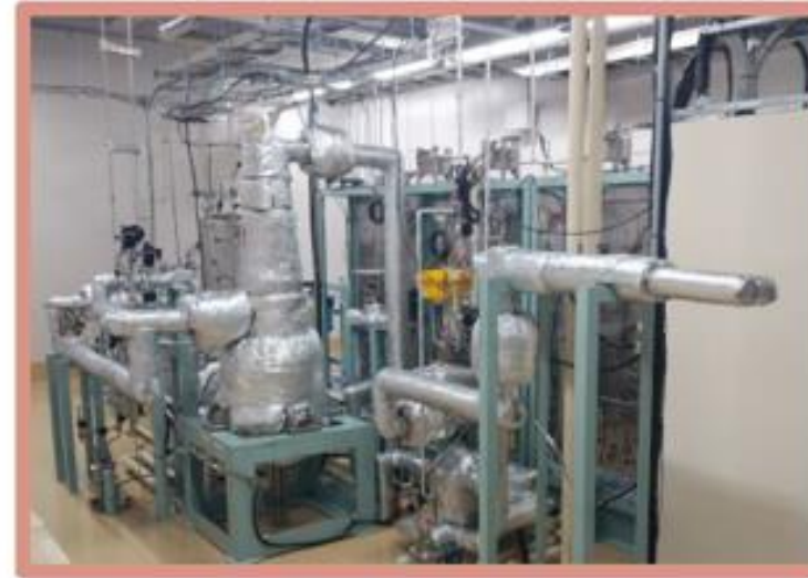
Flow accelerated corrosion test
